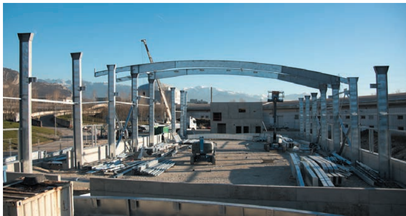
Fig. 6: The frame structure of the new assembly building ESRF 01 was put into place in December 2016.
