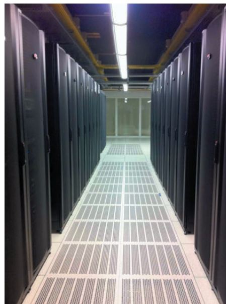
Fig. 4: New data centre in the central building.
